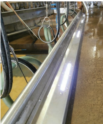
Work area illumination ensures better milking conditions.
